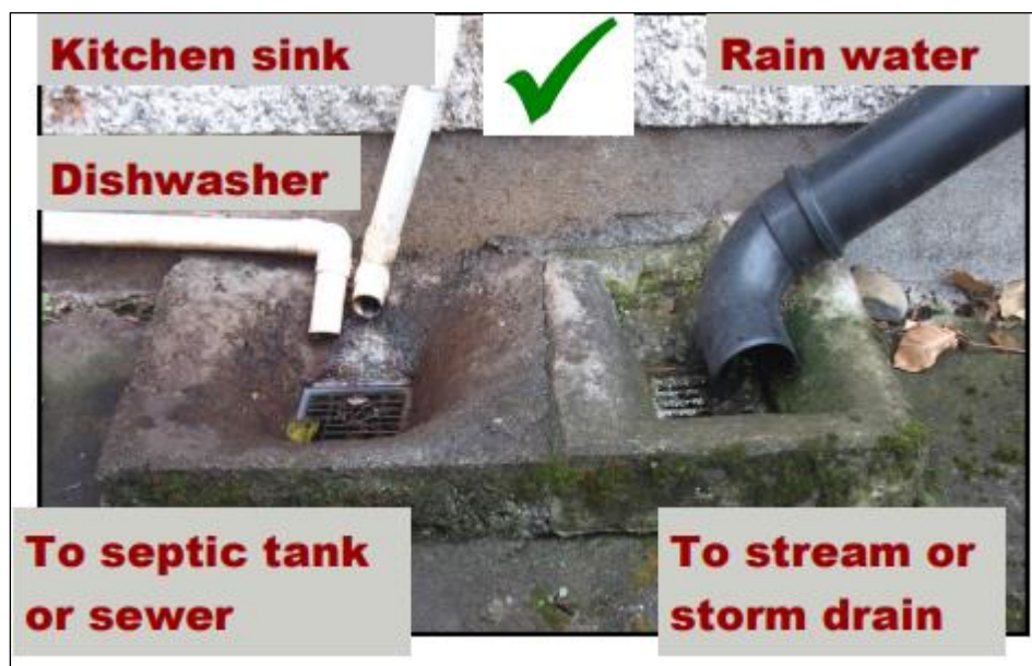
Figure 36. Correctly plumbed premises.
